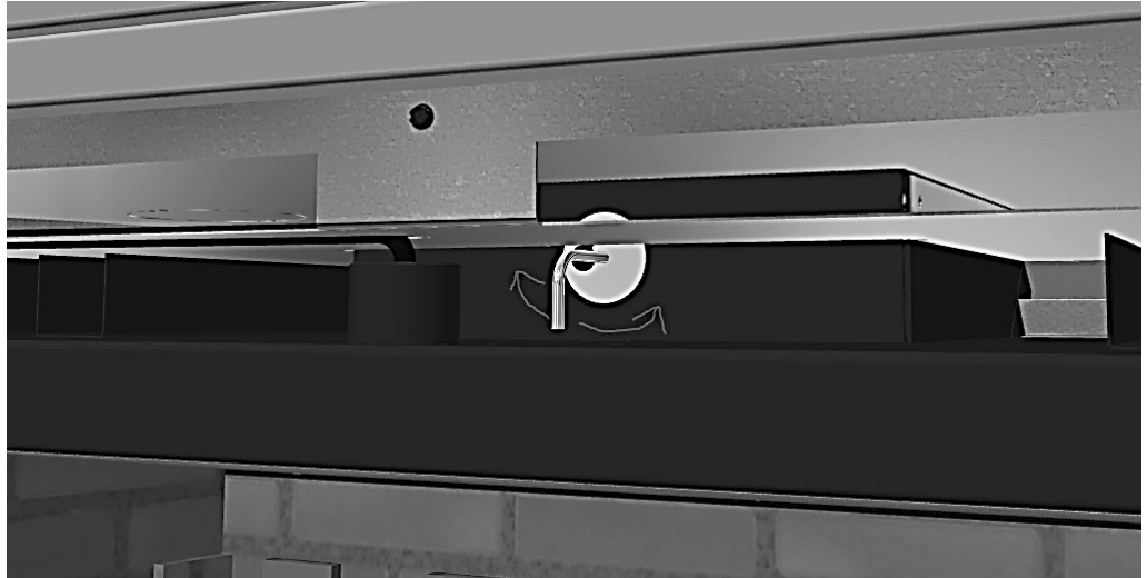
Figure 4-14 Exhaust Damper Adjustment
